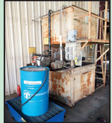
COOLANT PUMPING SYSTEM
