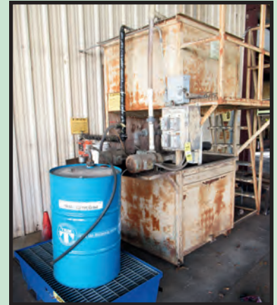
COOLANT PUMPING SYSTEM
