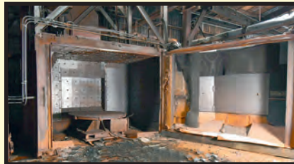
WHEELABRATOR 72" ROTARY TABLE SHOTBLASTING SYSTEM
