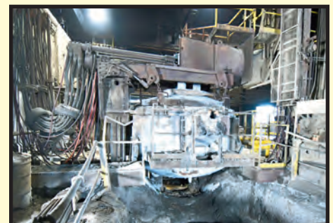
WHITING ELECTRIC ARC FURNACE
