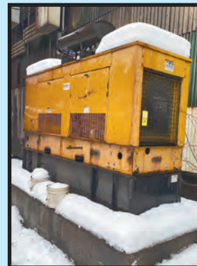
CATERPILLAR CD125-K366 DIESEL BACKUP GENERATOR SET
