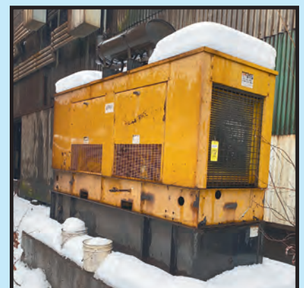
CATERPILLAR CD125-K366 DIESEL BACKUP GENERATOR SET
