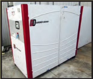
GARDNER DENVER VS70 100 HP AIR COMPRESSOR
