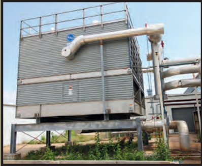
BAC COOLING TOWER
