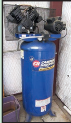
7 HP AIR COMPRESSOR
