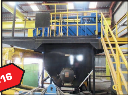
DEL CORP. DEWATERING SYSTEM
