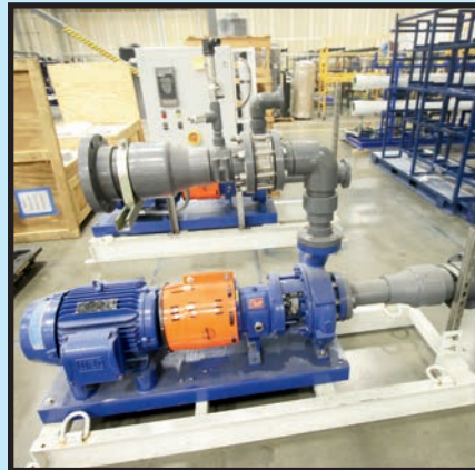
(2) TITAN CENTRIFUGAL PUMPS – 40 HP, 15 HP
