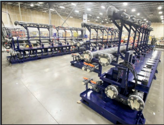
(3) MI SYSTEMS FILTRATION SKIDS – ARCA WORK IN PROCESS
