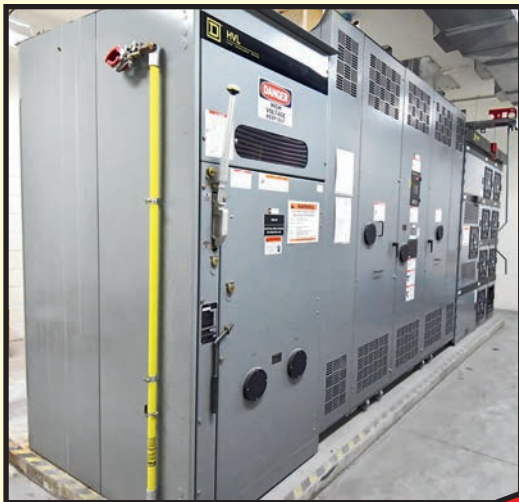
HIGH QUALITY SWITCHGEAR
