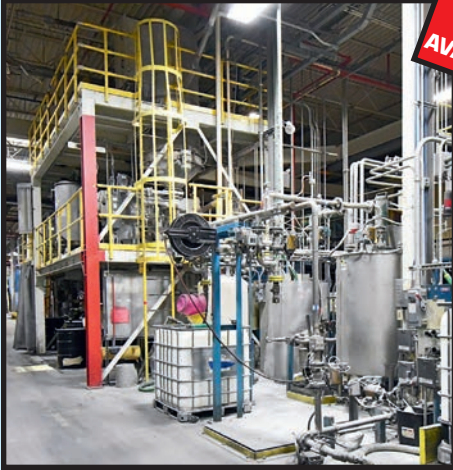
STAINLESS MIXING AND STORAGE SYSTEM
