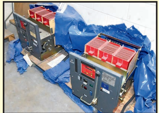
NEW CIRCUIT BREAKERS
