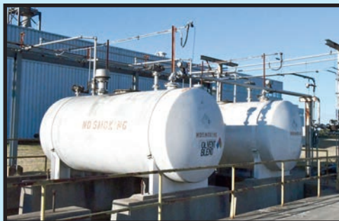
SOLVENT TANK SYSTEM
