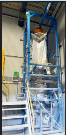
SUPER SACK UNLOADER AND WEIGH FEED HOPPER
