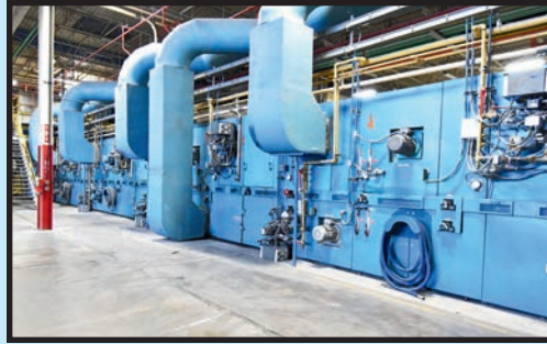
BRUCKNER 12-ZONE GAS FIRED BELT OVEN
