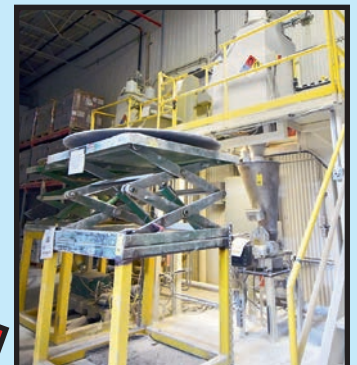
MATERIAL BINS W/WEIGH HOPPERS
