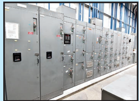
HIGH QUALITY SWITCHGEAR
