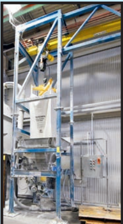
SUPER SACK UNLOADER W/BIN, BLOWER AND 6-POSITION CRANE SYSTEM
