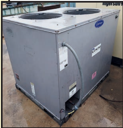
CARRIER COMMERCIAL CONDENSING UNIT
