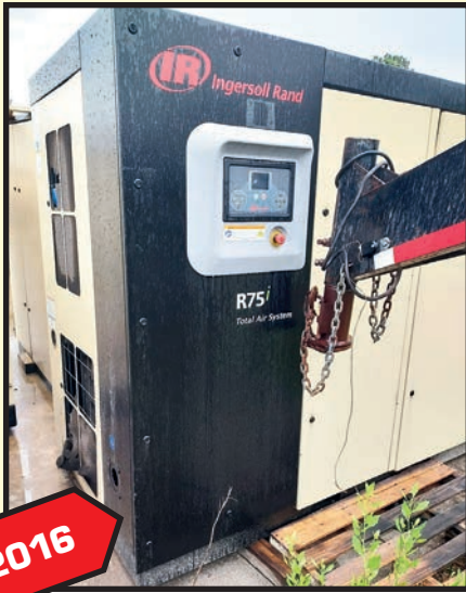
INGERSOLL RAND 100 HP ROTARY SCREW AIR COMPRESSOR
