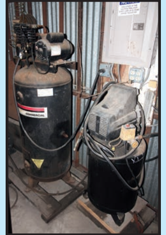
VERT. AIR COMPRESSOR
