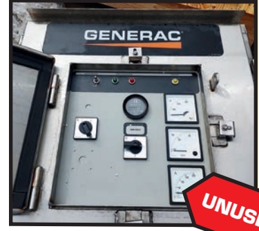
(1 OF 2) GENERAC AUTO. TRANSFER SWITCHES
