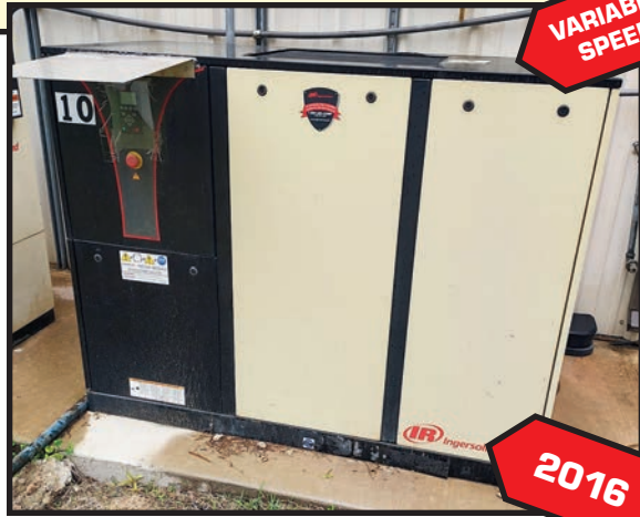
INGERSOLL RAND 25 HP ROTARY SCREW AIR COMPRESSOR
