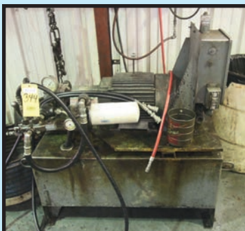
HYDRAULIC TEST UNIT
