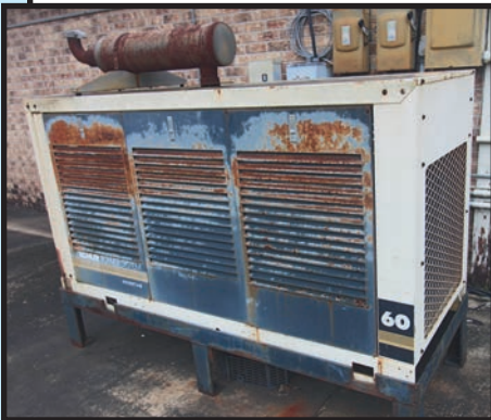
KOHLER BACKUP GENERATOR
