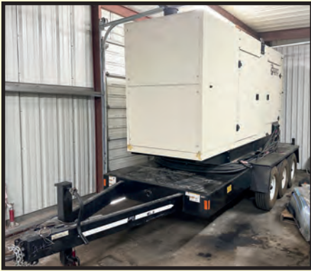
TRITON 350 KW BACK UP GENERATOR
