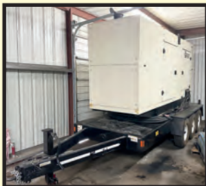
TRITON 350 KW BACK UP GENERATOR
