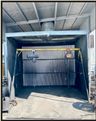
OPEN SIDED REAR DRAFT PAINT BOOTH
