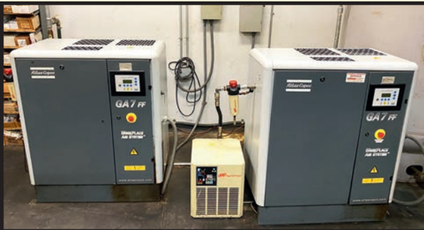
(2) ATLAS COPCO GA7-FF ROTARY SCREW AIR COMPRESSORS
