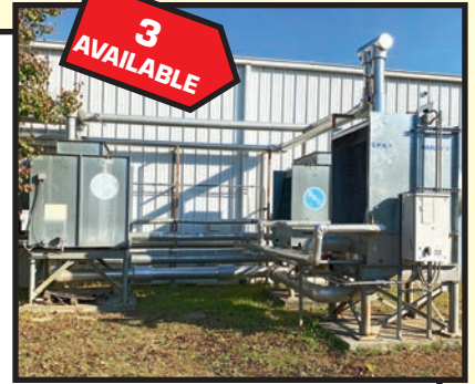
BAC & MARLEY COOLING TOWERS
