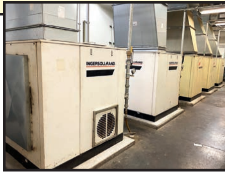
(5) INGERSOLL RAND ROTARY SCREW AIR COMPRESSORS
