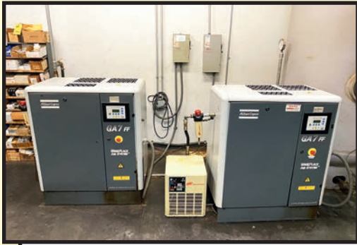
(2) ATLAS COPCO GA7-FF ROTARY SCREW AIR COMPRESSORS
