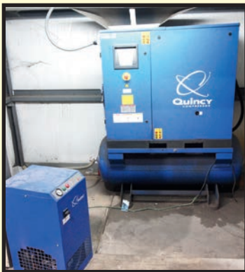
QUINCY 20 HP ROTARY SCREW TYPE AIR COMPRESSOR AND DRYER
