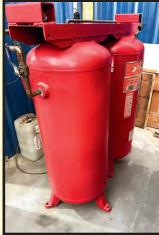
(2) HUSKY 60 GAL. RECEIVING TANKS
