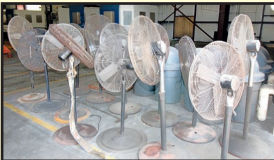
SAMPLE VIEW OF SHOP FANS
