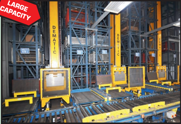
DEMATIC AUTOMATIC STORAGE AND RETRIEVAL SYSTEM
