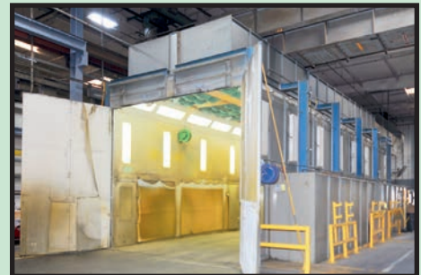
BINKS DRIVE-THRU PAINT SPRAY BOOTH
