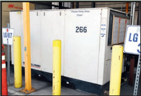
INGERSOLL RAND 150 HP ROTARY SCREW AIR COMPRESSOR
