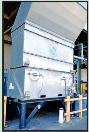
BALTIMORE AIR COIL COOLING TOWER
