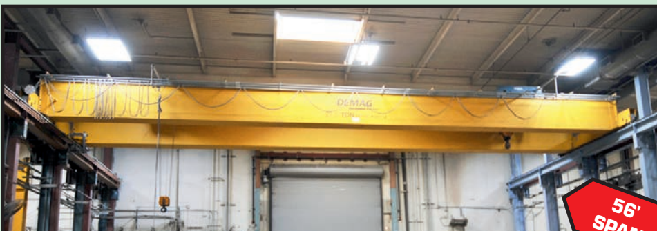
DEMAG 27.5 T. OVERHEAD BRIDGE CRANE
