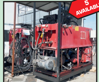
NOV HYDRAULIC POWER SUPPLY
