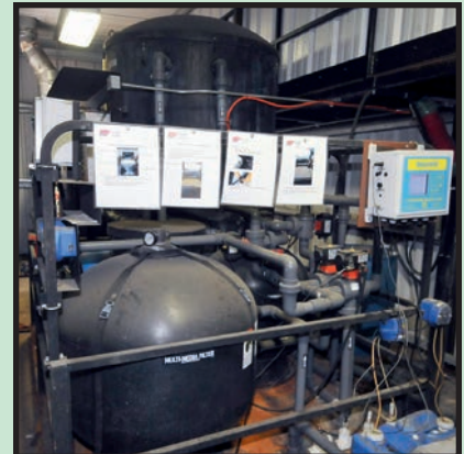
WATER MAZE WASTE TREATMENT SYSTEM
