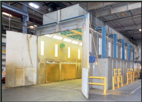
BINKS DRIVE-THRU PAINT SPRAY BOOTH
