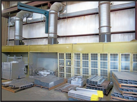
SPRAY PAINT WALL EXHAUST SYSTEMS
