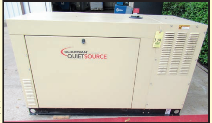
GENERAC GUARDIAN QUIET SOURCE GENERATOR
