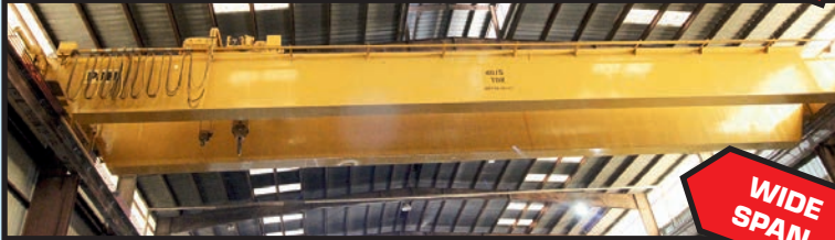
P&H ENGINEERING 40 T. X APPROX. 90' SPAN OVERHEAD BRIDGE CRANE
