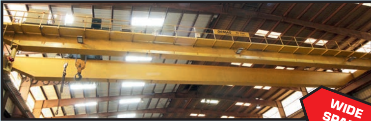
DEMAG 40 T. X APPROX. 109' SPAN OVERHEAD BRIDGE CRANE
