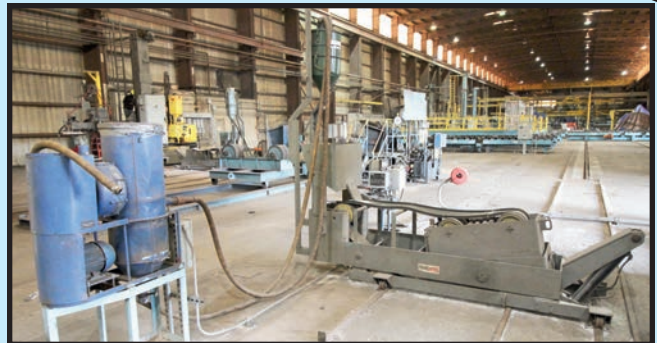
PANDJIRIS CONVEYOR STYLE FLUX RECOVERY HANDLING SYSTEM
