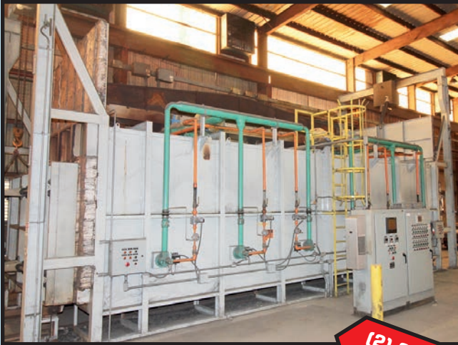
ENERGY SERVICES GROUP CAR BOTTOM FURNACE
